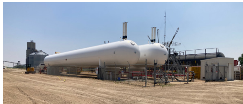
A 90,000-gallon propane storage tank will be added to the Welcome propane terminal this fall.
