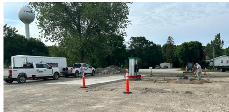
At Thompson, we excavated the parking lot, poured a new diesel island, and installed new lighting.
